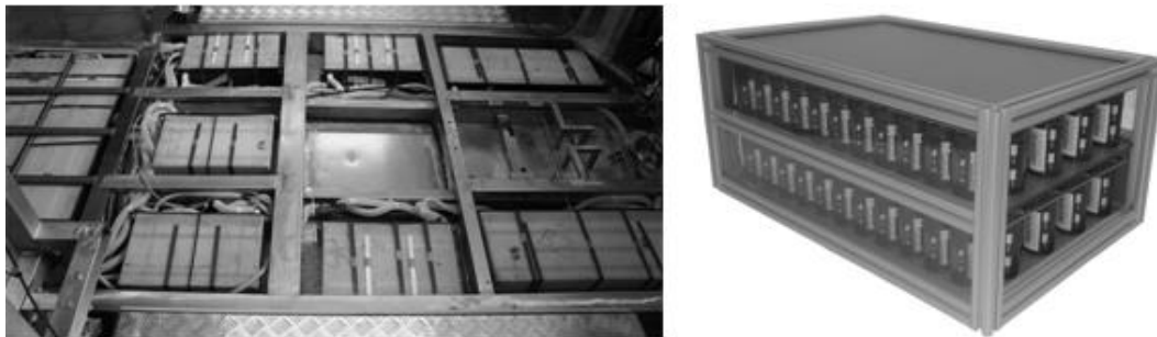
Fig. 3.1. Electrochemical battery pack placed in the chassis (left) and ultracapacitor energy storage (right)
